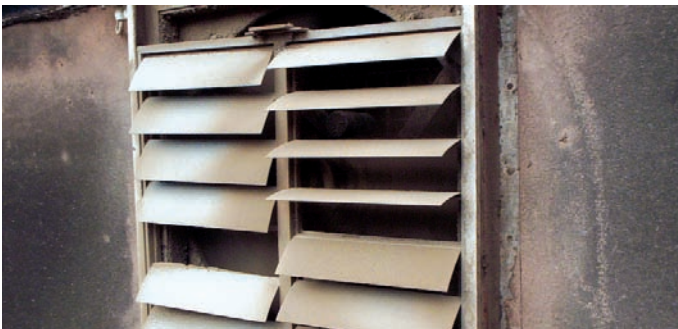
Broken flaps are a common maintenance fault
